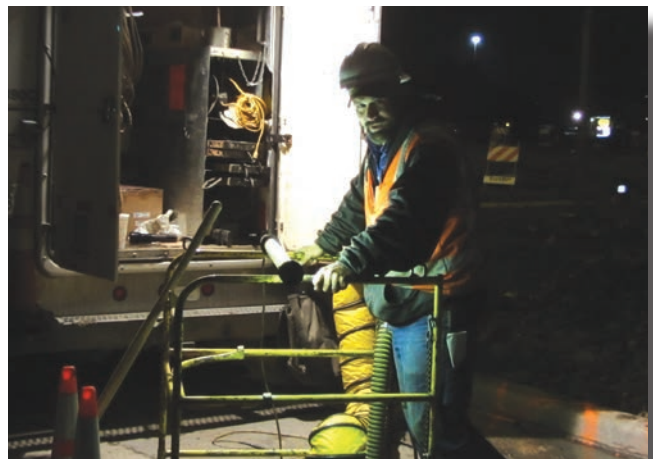
Paul Cavenaile work an all-nighter repairing a 900-pulp cable hit at 75th & Lemont Road.
